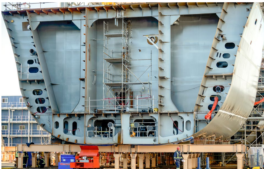
Seaspan continues to make great progress on its fourth vessel, the first of two critically important Joint Support Ships
